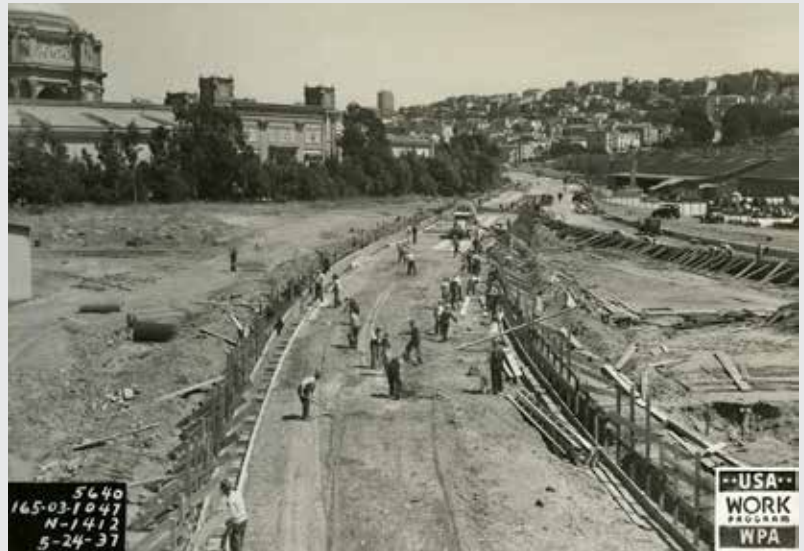
View of WPA crews at work on the Lyon Street approach to the Golden Gate Bridge, May 24, 1937. Photographer unknown, Work Projects Administration, San Francisco, California.
